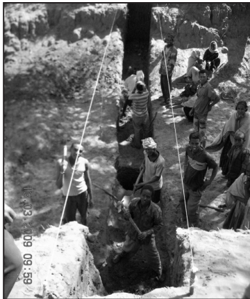
Fig. 5 | Construction site of the subsurface dam Koraro-01 during digging of the trench for the clay sealing wall (Foto: KLOPPER 2009)
