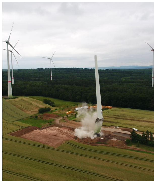
Fig. 1: Execution of a tower demolition using the folding blast method. Using a second explosive charge at 1/3 of the total height, the upper part of the tower collapsed in the opposite direction to the lower part. This method is more space-saving than a conventional tower collapse blasting. © Reisch Sprengtechnik GmbH
