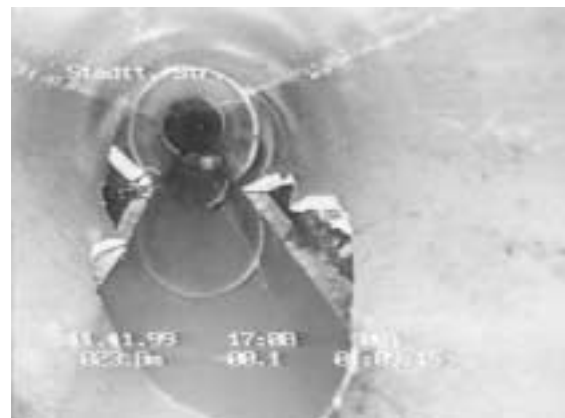
Figure 14. Parts of the invert missing
