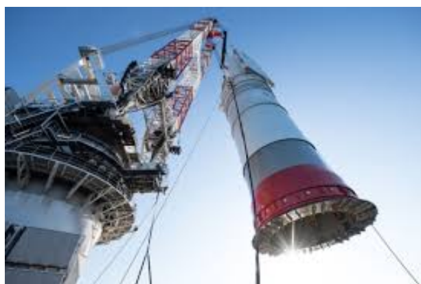
Fig. 4: IHC noise mitigation system, © Ørsted.
